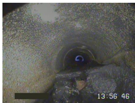
...deposits at the bottom of the pipe
