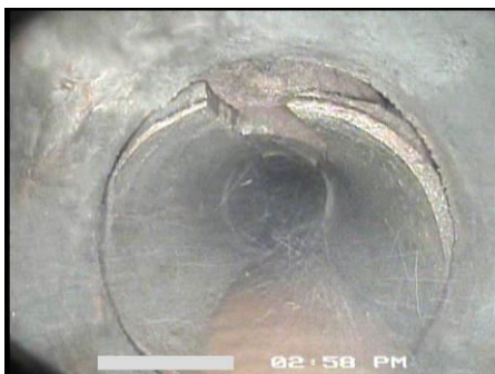
...localized pipe damage
