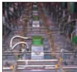
MasterCooler SMART® in slab plant
